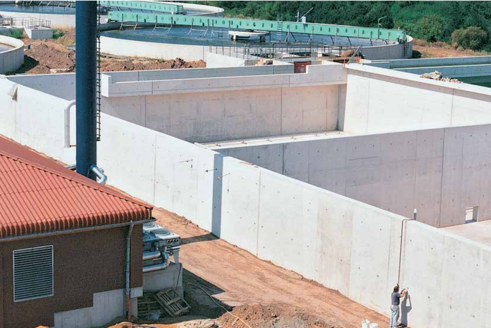
Sewage works in Hameln, Germany.
